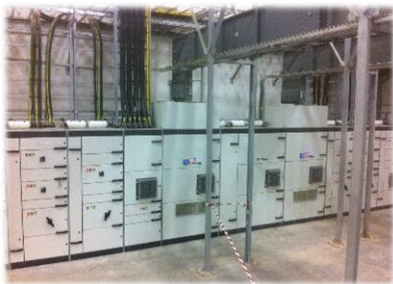
Fig. 6 – R-DLP system with white extinguishant storage cylinders in a Saudi Arabian electrical substation.
