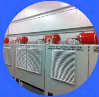
Electrical cabinets with DLP System.
