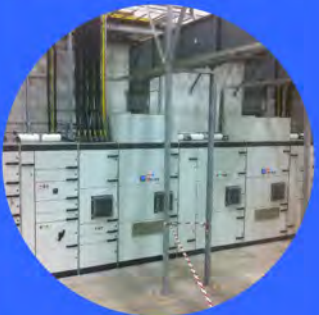
Sub-Station & white DLP agent cylinders
