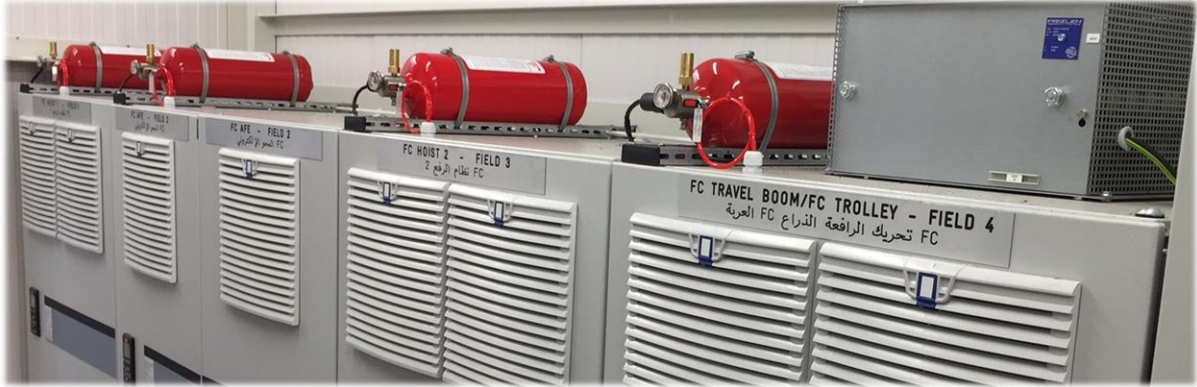
Fig. 1 R-DLP system protecting against fire in electrical control room switchgear of exported shipping container crane.
